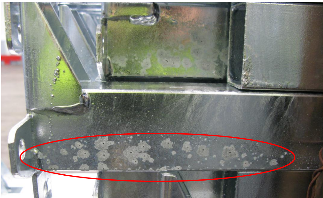
White rust on 60x40 post. Approved appearance according to EN ISO 1461:2009.
